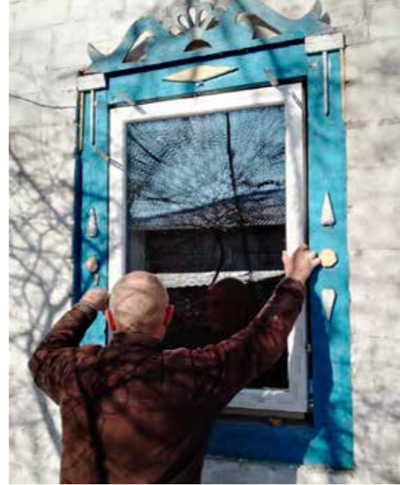
Above: One of the most common repair tasks that arche noVa facilitated in Ukraine in 2023: replacing destroyed windows.
