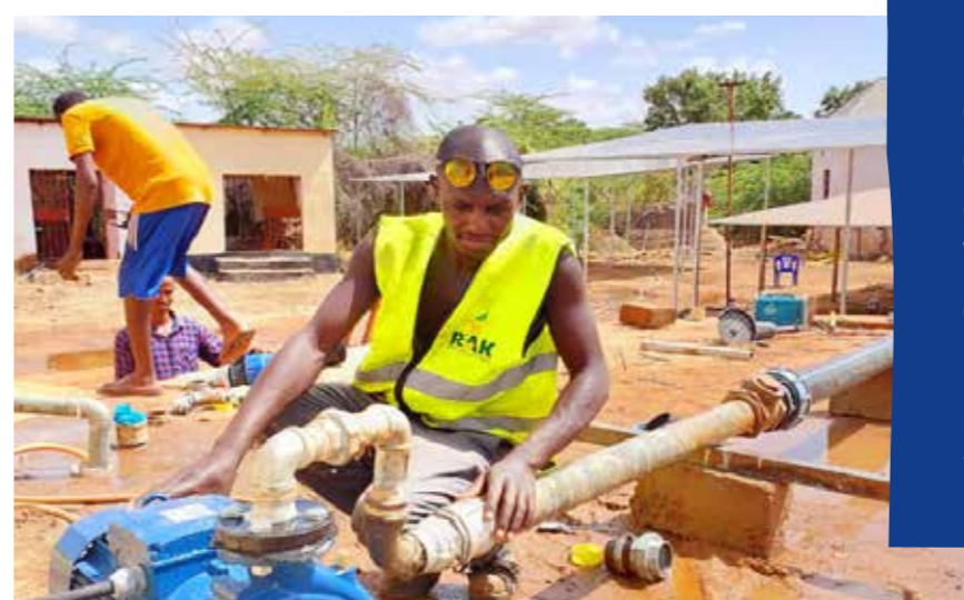
Below: In expanding water supply systems like in Belet Xawoo in the Gedo Region (Jubaland), solar power systems are being installed for energy provision.
