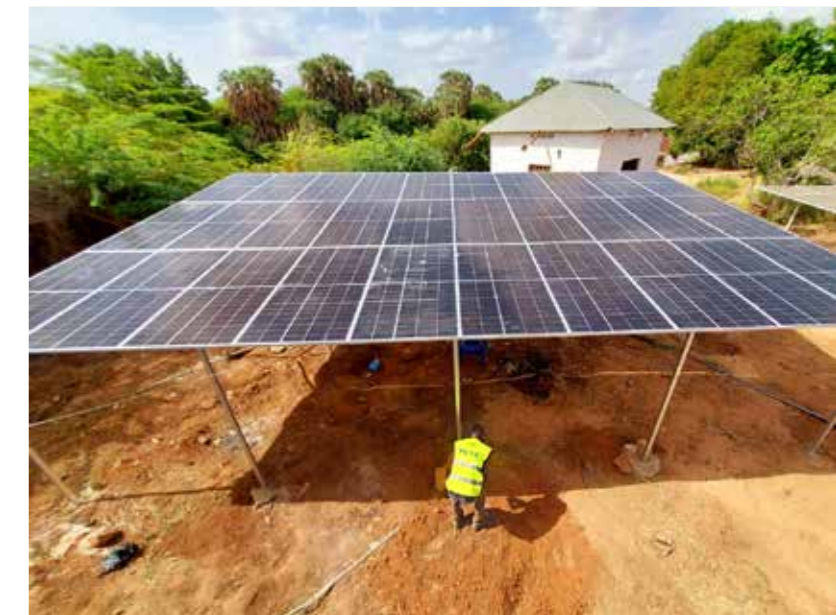
Solar technology as an energy source for water supply systems, as seen in this image from Somalia, is a step towards greater sustainability in arche noVa's work. This approach is actively promoted by the Board.
